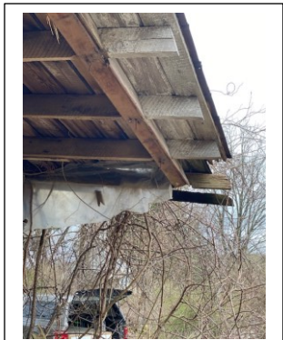
The Barn Roof Hanging over the road
